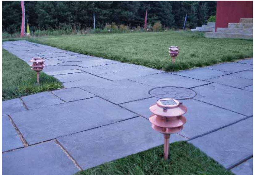
Temporary solar footpath lights help illuminate the khora path around the Gonpa at Padma Samye Ling.
